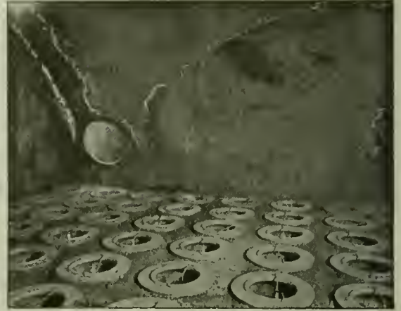
Interior of High Tension, Direct Current, Electrode Chamber Inside of Flue Tube Measuring 13 Feet in Diameter. The Electrodes Are Suspended Chains Which Carry the Charge When in Use.
